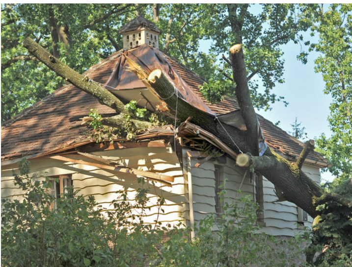
Damage from June 2012 derecho storm.
